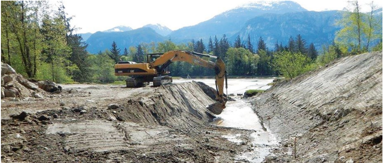
Construction preparing for the new box culverts. (Credit: Squamish River Watershed Society)
