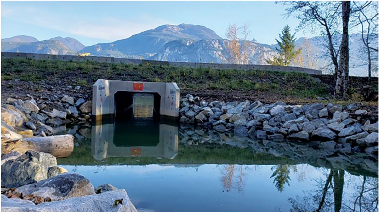
A box culvert installed in the dike to increase connectivity between the Squamish River and the estuary. (Credit: Edith Tobe)
